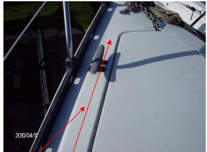
B2 Elevated moisture meter readings where tested at random suggest water intrusion.
