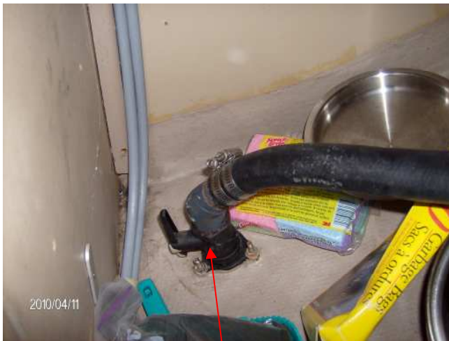
B3 fitting loose here
