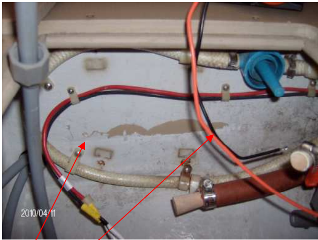
B1 tabbing failure here to here
