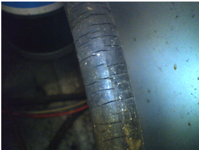
B7 fuel supply hose deteriorated
