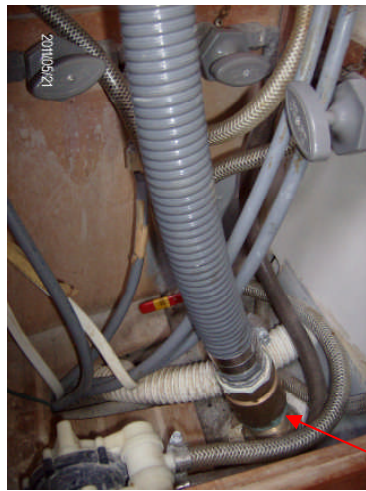
B3 galley sink drain thru hull fitting is loose in the hull
