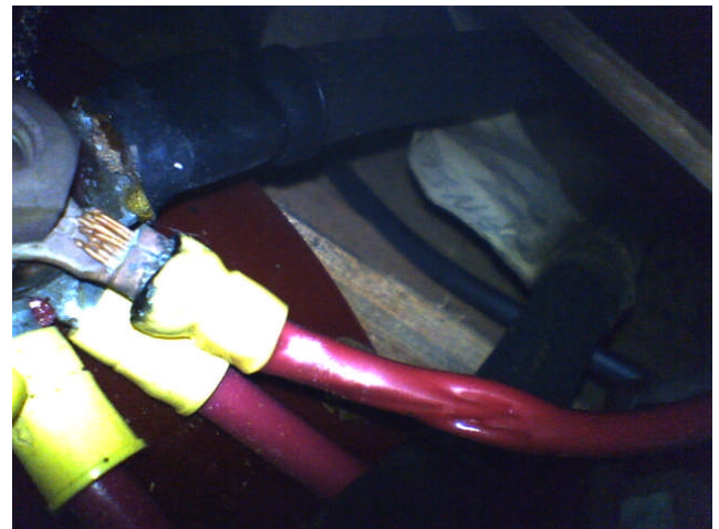
B8/3 burnt wiring behind the 12-volt DC
