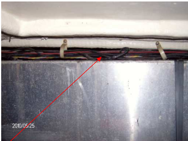
B4 12 volt DC wiring laying on top the fuel tank
